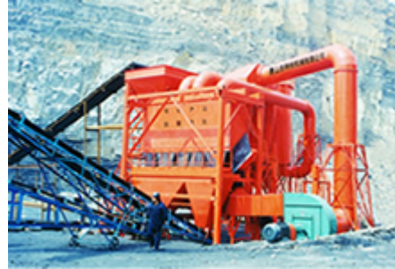
Air cleaning system Source: http://www.tsganxuan.com
